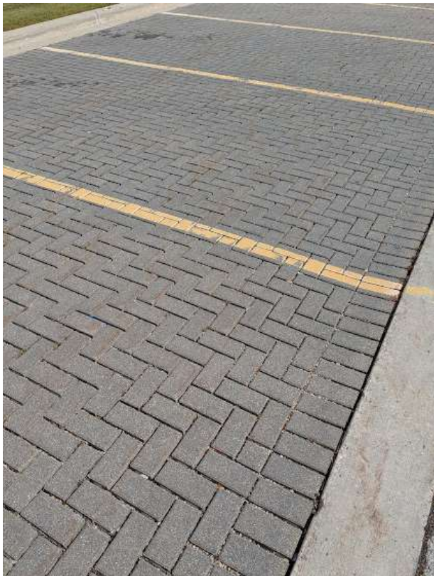
CVS pharmacy in Sturgeon Bay has a section of their parking lot composed of these pavers.
